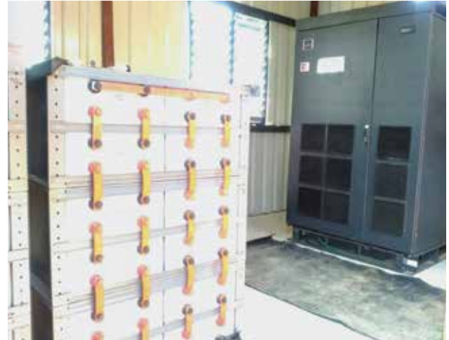
VRLA Battery Bank
