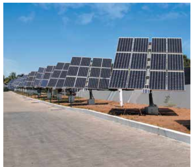
Jain Solar Pumping System
