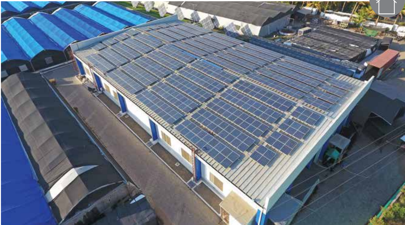
Solar Roof Top Grid Connected Plant
