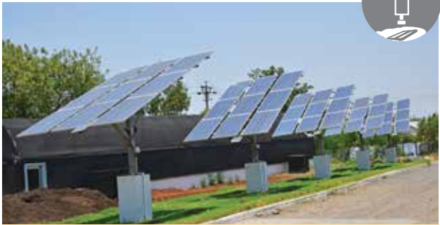
Jain Solar Pumping System
