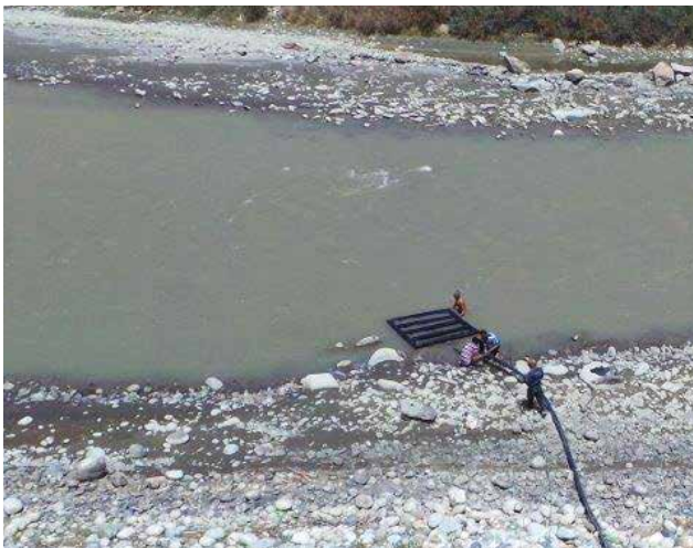
Floating Submersible Pump in Indus River
